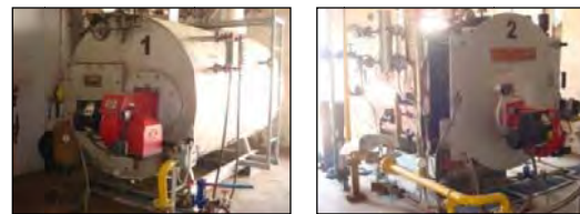
Gambar 1. Boiler #1 dan Boiler #2 PT. Textile Industry
