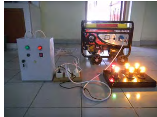
Figure 10. Photograph of ATS loading test using incandescent lamps, electricity from PLN network and portable generator available at the same time.
