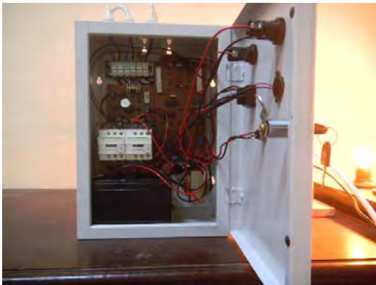
Figure 8. Photograph of assembled automatic transfer switch inside panel box
