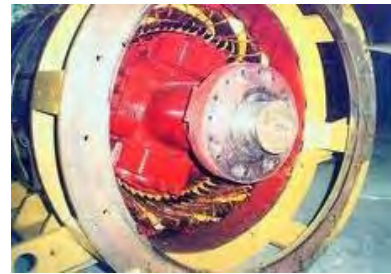
Gambar 3. Stator Coil Generator
