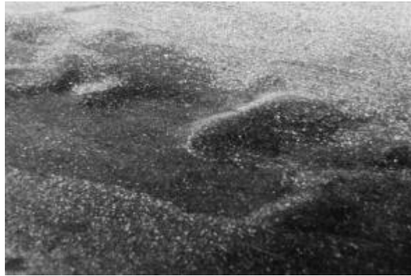
Gambar 2. 14 Kerusakan Sungkur (Shoving)
