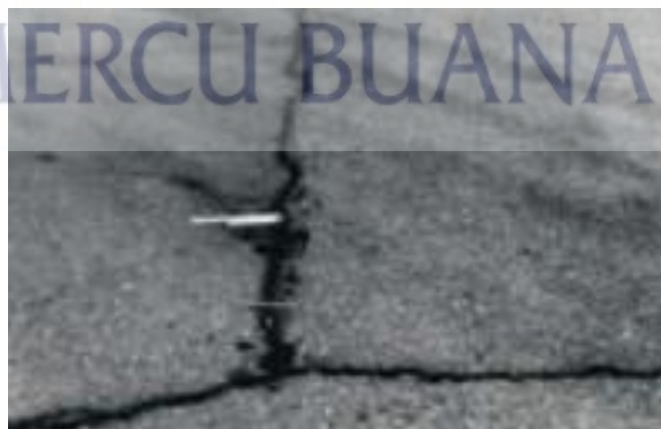
Gambar 2. 9 Retak Refleksi Sambungan ( Joint Reflection Cracking )
