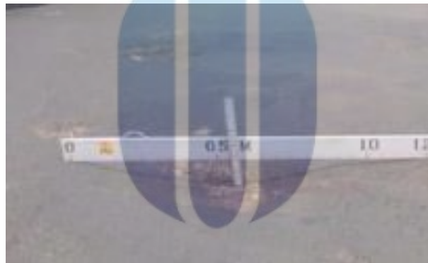
Gambar 2. 7 Retak Amblas ( Depression )
