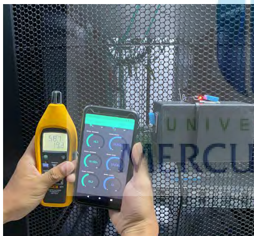
Figure 4 Temperature and Humidity Sensors testing on the Cold Air
