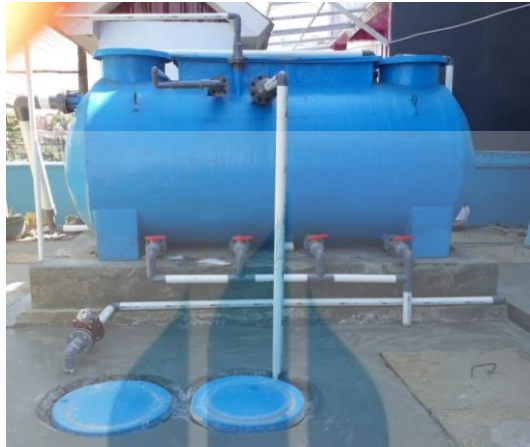
Gambar 4.15 Sewage Treatment Plant
