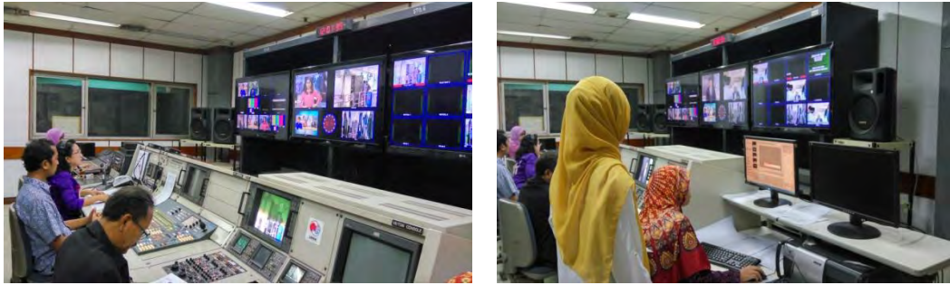
Ruang Sub Control
