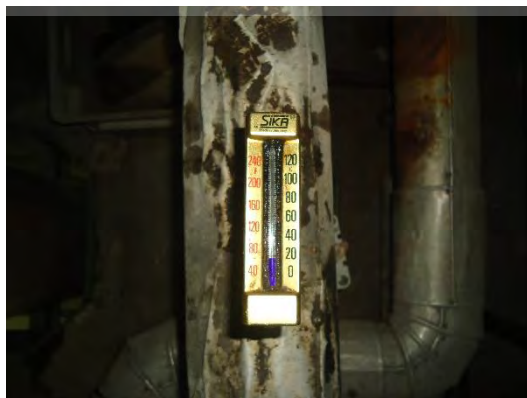
Gambar 2.6 Termometer Cooling Coil
