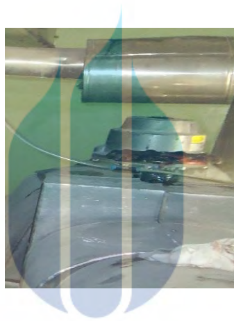
Gambar 2.13 Valve Pengatur Chiller Pressure
