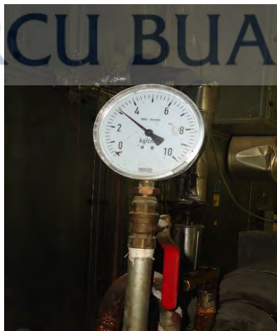
Gambar 2.14 Pressure Gauge Chiller
