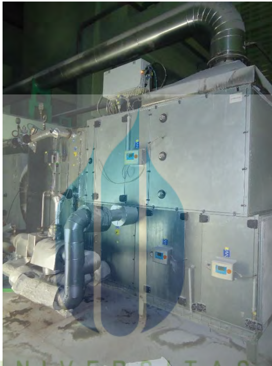
Gambar 2.3 Air Handling Unit
