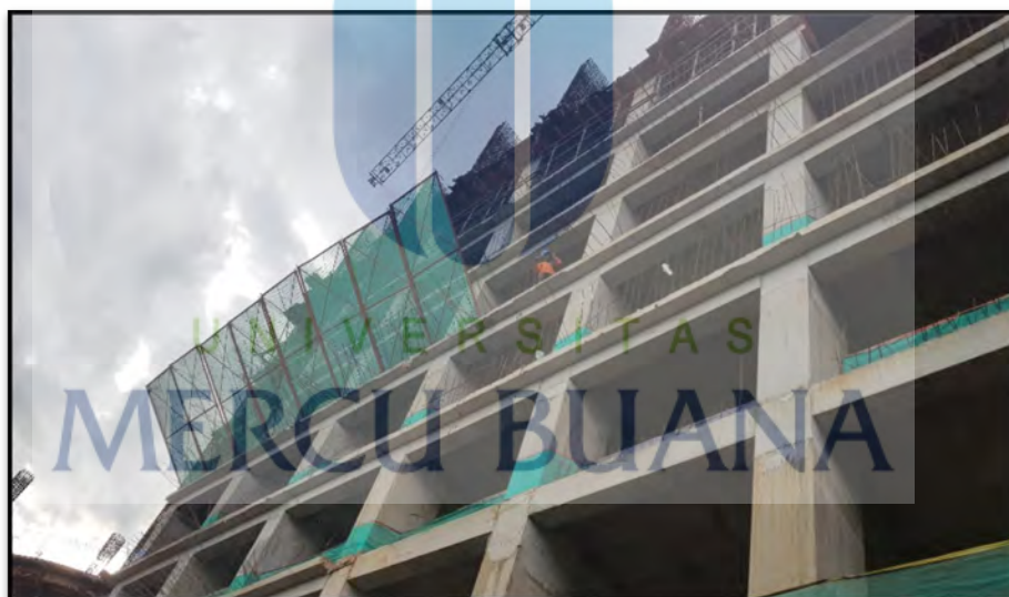
Gambar 6.18 Safety Deck dan Safety Net
