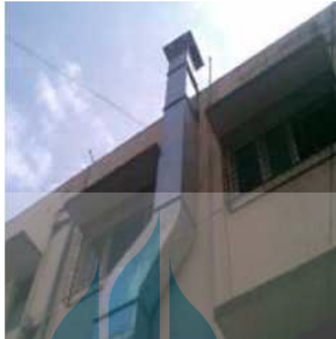
Gambar 2.7. Exhaust Air Ducting
