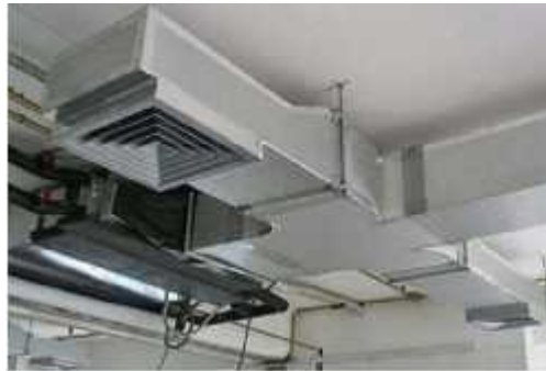
Gambar 2.5. Supply Air Ducting
