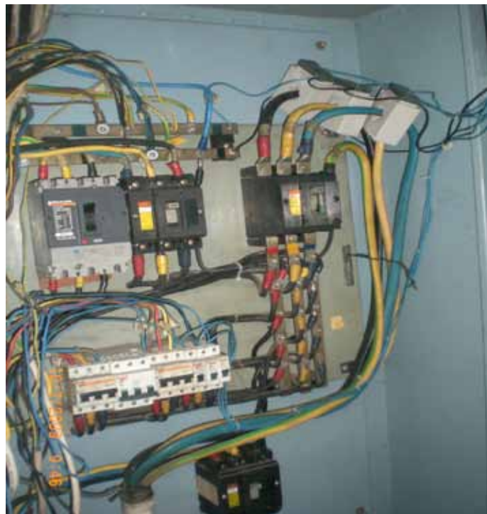
Gambar 6.29 Panel power dan penerangan DIDCL1G2
