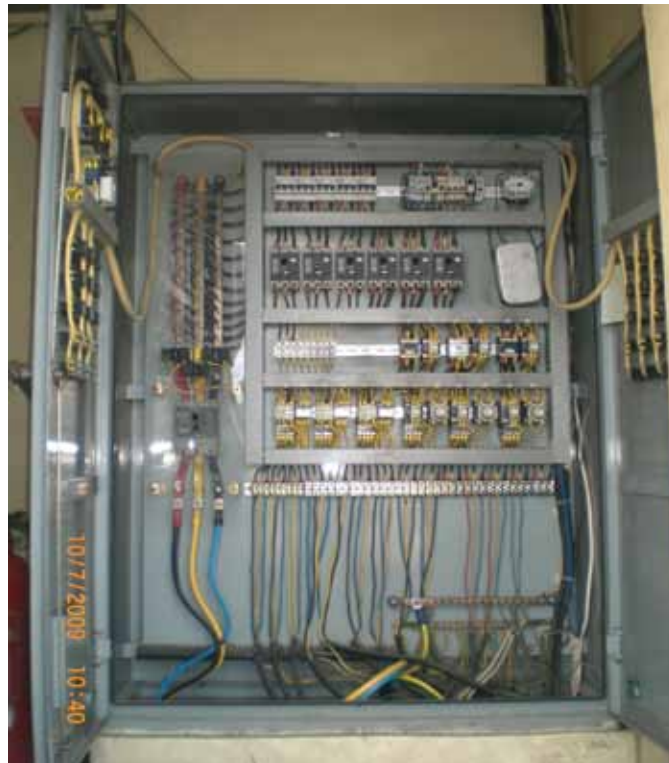
Gambar 6.25 Panel power cooling tower L9G1
