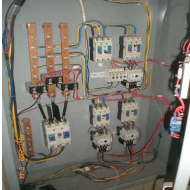
Gambar 6.28 Panel power pompa artesis L1G1
