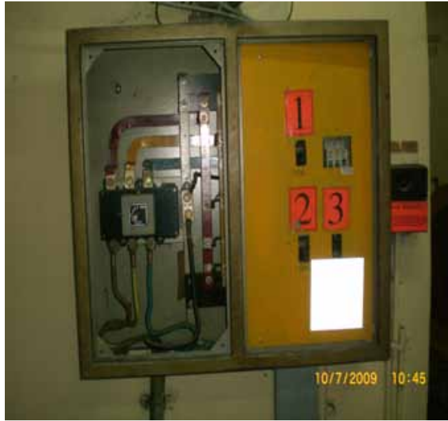
Gambar 6.26 Panel power lift L9G1
