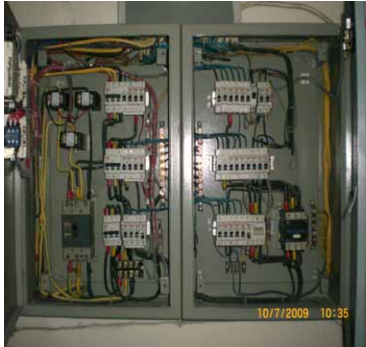
Gambar 6.8 Panel power dan penerangan L1G1
