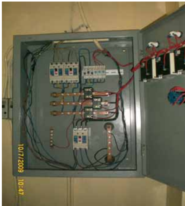
Gambar 6.27 Panel power pompa hydropoor L9G1
