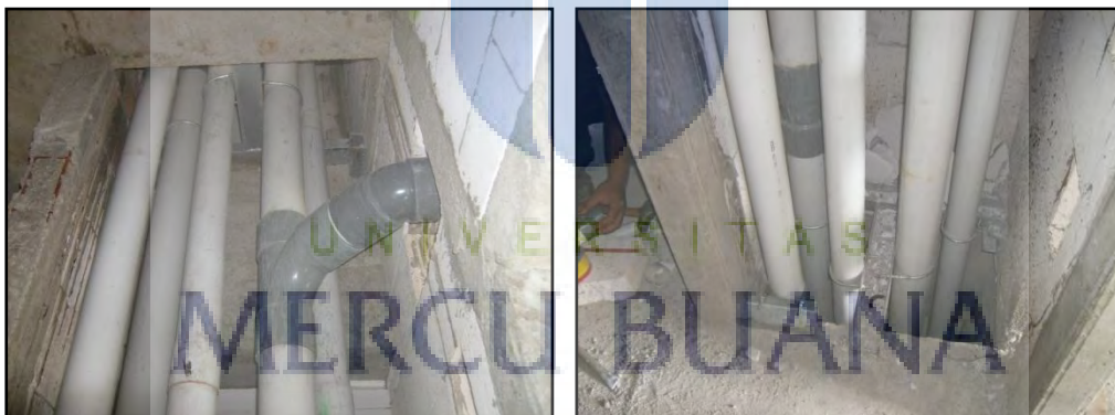
Gambar: Pipa plumbing
